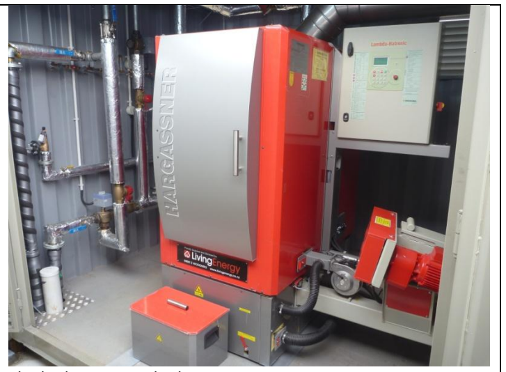
The boiler unit inside the container
