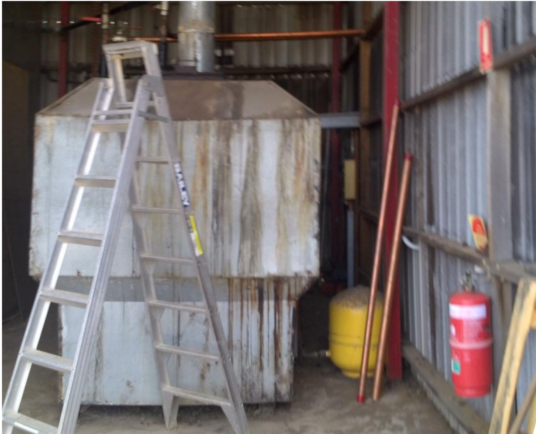
Figure 4: Photo of the timber kiln boiler
