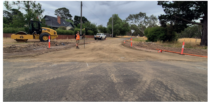
Design & Projects Engineer Memphis Forte checks progress on the Waubra-Talbot Rd works.
