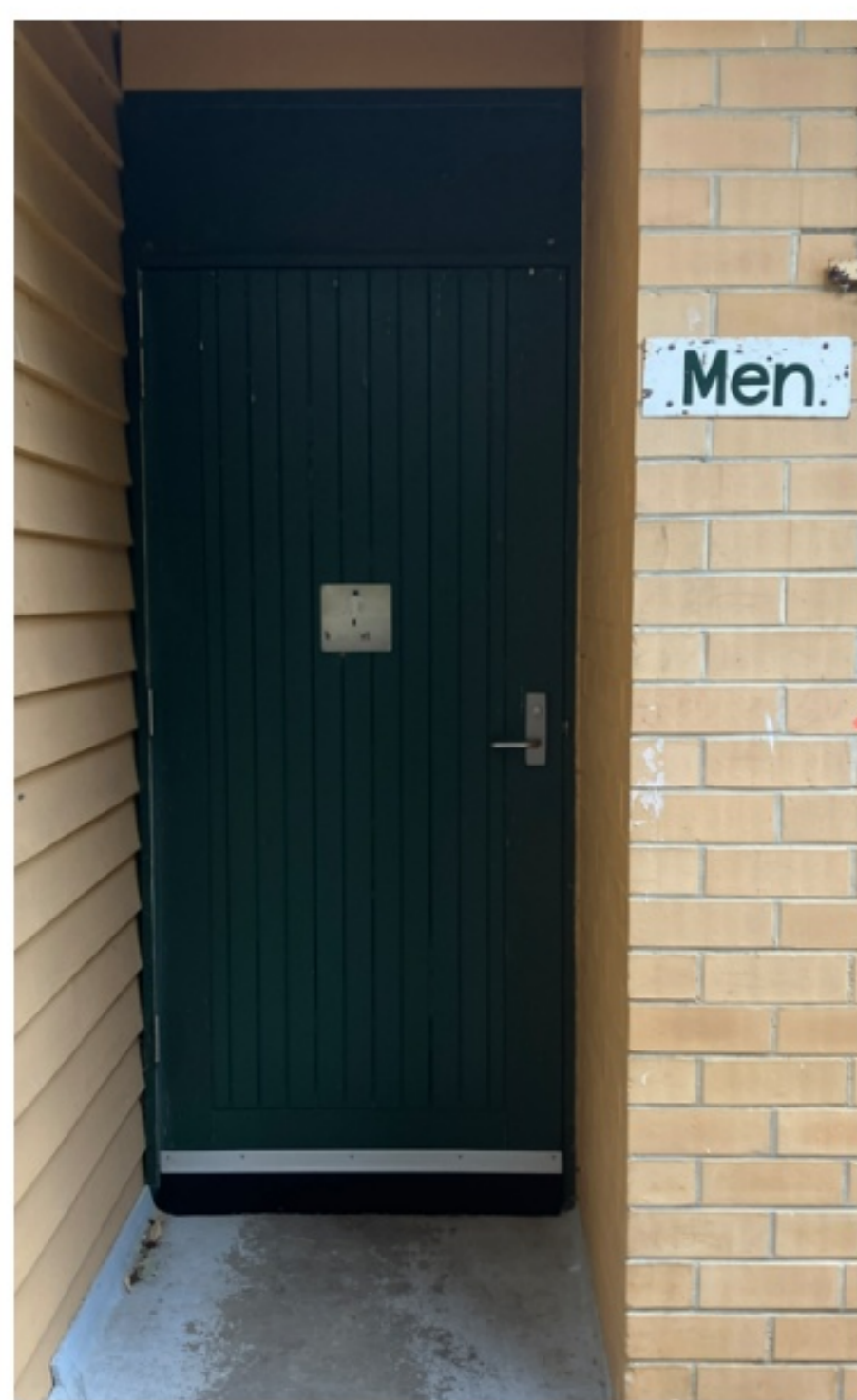
c. Entry Door: Paint and signage faded
