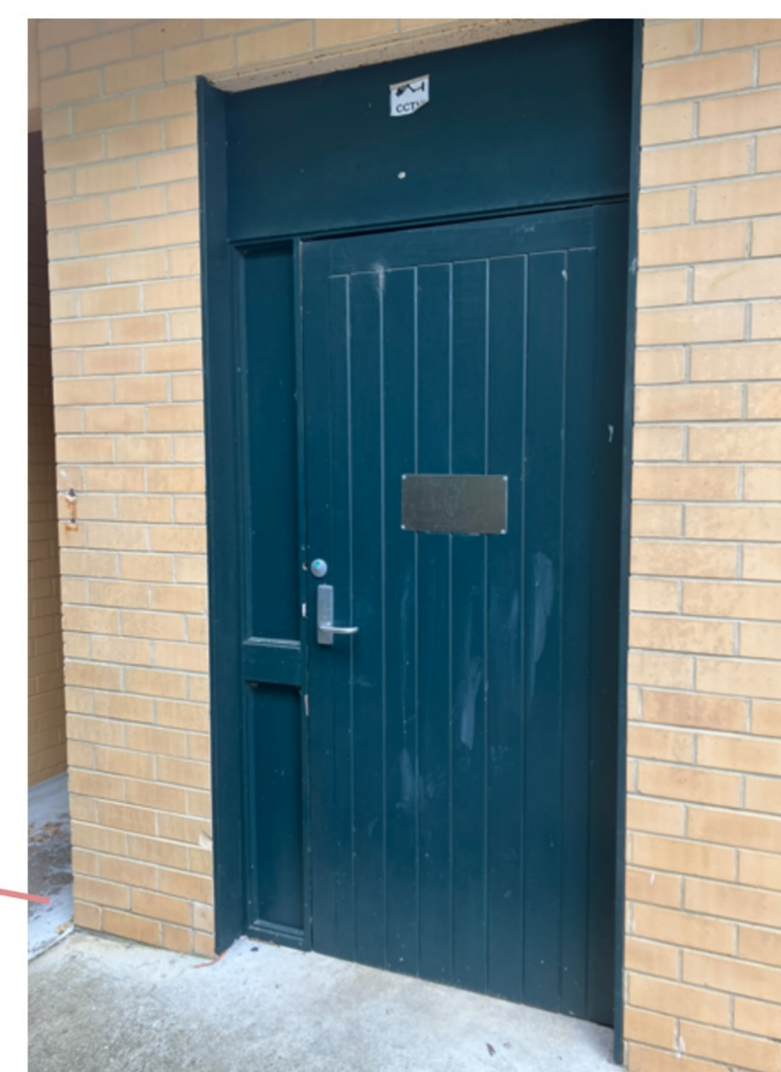
Faded entry door signage and paint on entry door
