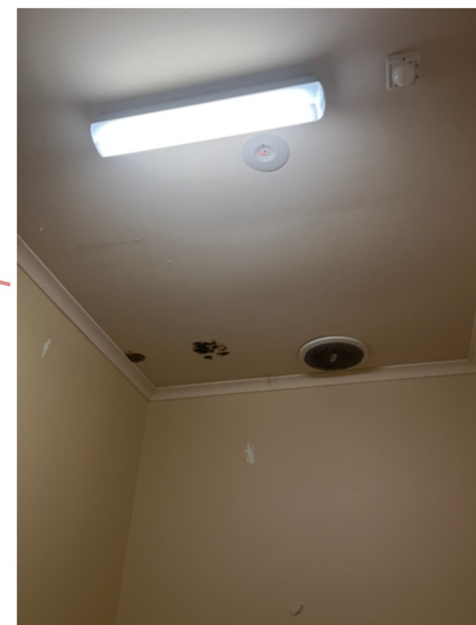
Black mold / water damage on ceiling
