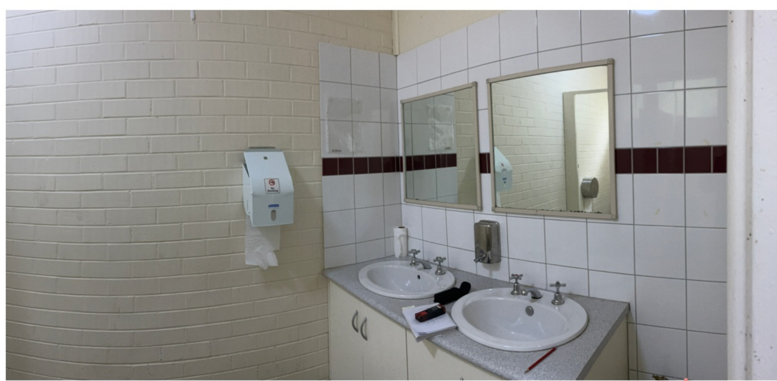
Wall finishes discolored; sanitary fixtures (drier and washbasin) are dated.
