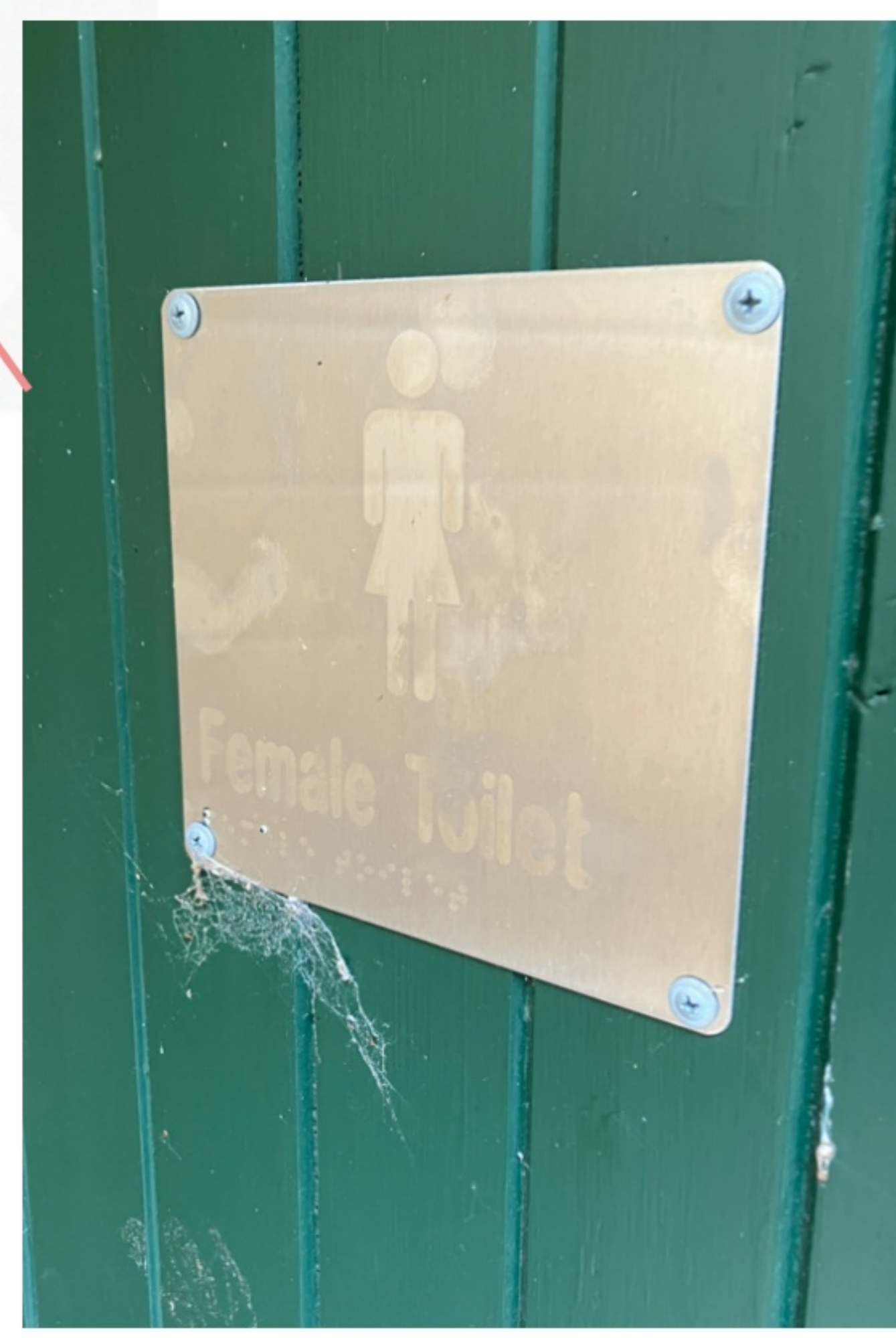
Entry door signage: Faded
