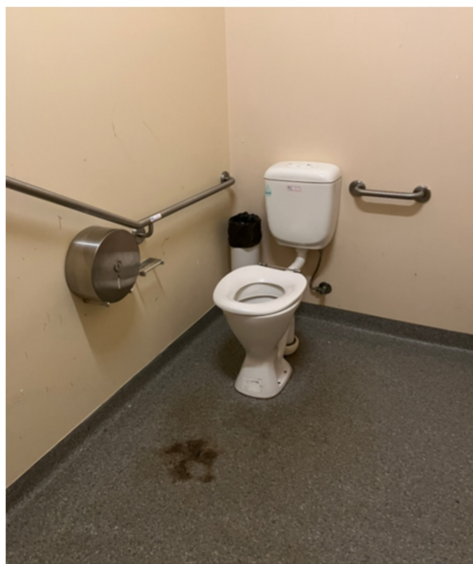
Staining on vinyl floor and dated toilet pan
