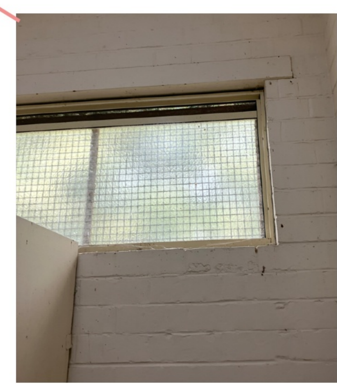
Timber Window deteriorated due to age
